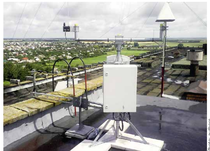
FIG 3 A tripod can be used to easily install the R&S®UMS100 monitoring systems on the flat roof of a tall building.
