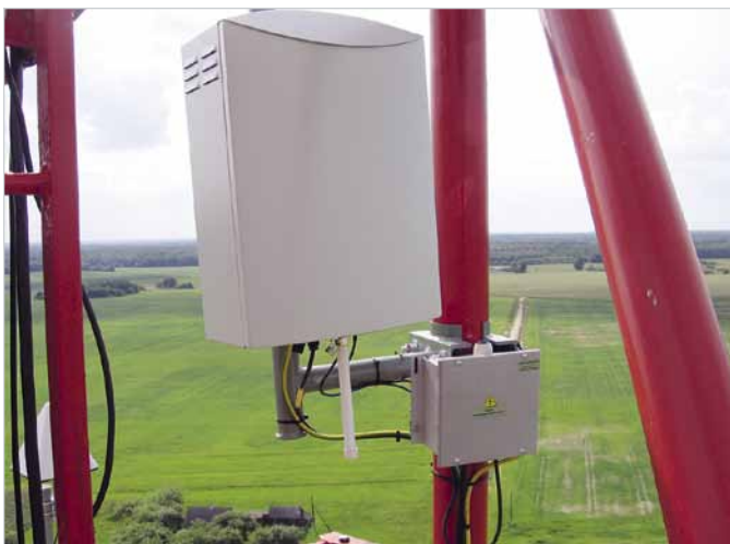
FIG 2 In this example, an R&S®UMS100 monitoring system is mounted on the mast of a mobile radio operator.
